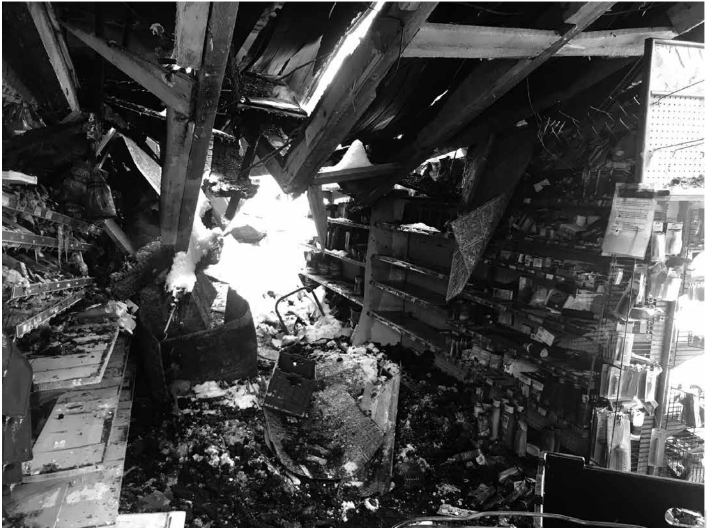
Interior photo of the damage from the Keene Valley Grocery fire.
